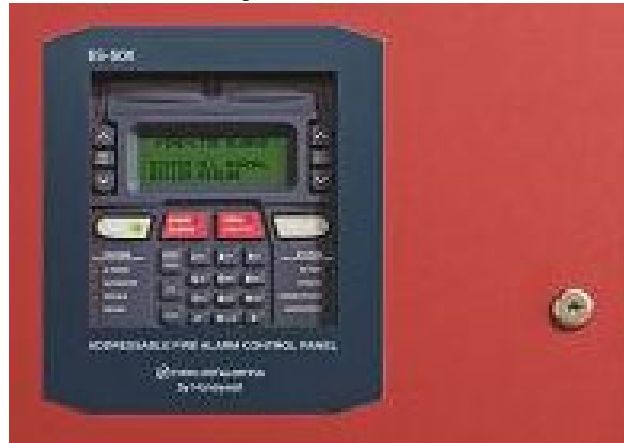
Figure 1 - Honeywell Addressable Fire Alarm Control Panels ES-50X
