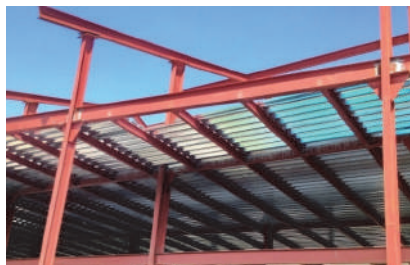
Fig.1 - Example of the device of the building frame using composite steel and concrete structures.
